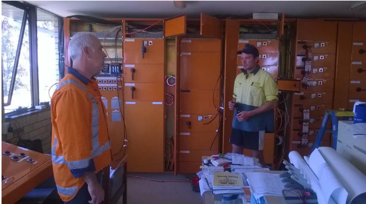
Telemetry board being stripped and rewired in advance of the new telemetry program implementation. Left: Project Coordinator-Simon Cartwright, Southern Cross Consulting Right: Project Electrician – Mark Notley, ETE Services
